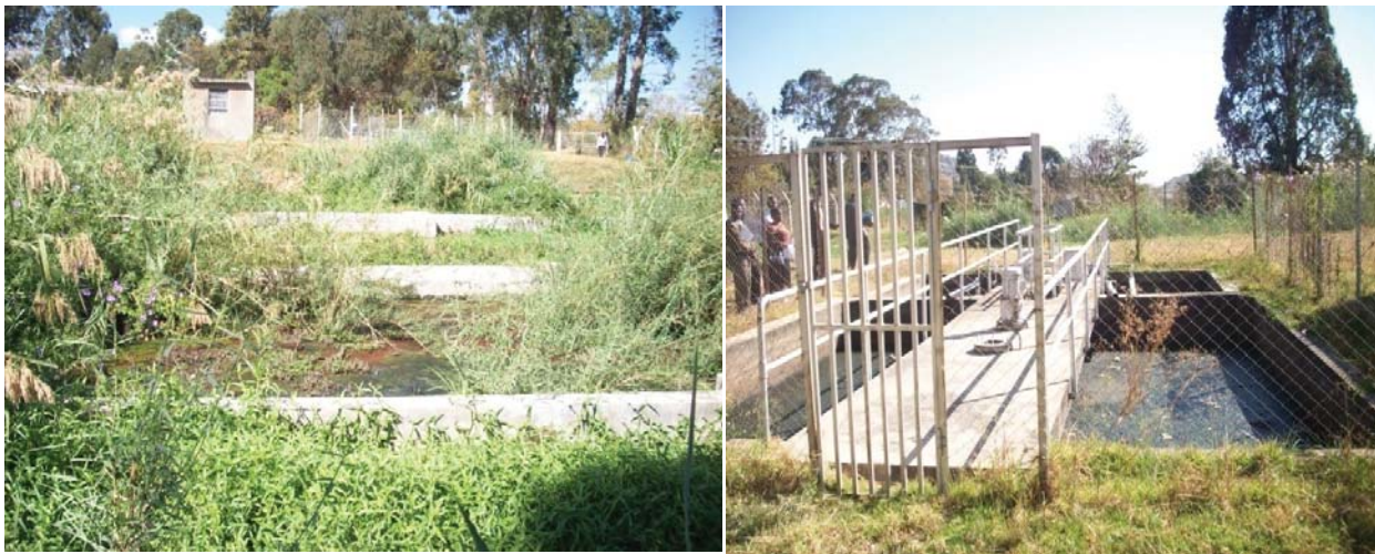
Plate 6: Constructed Wetland and Mechanical Aeration Chamber at Kleruu TTC
