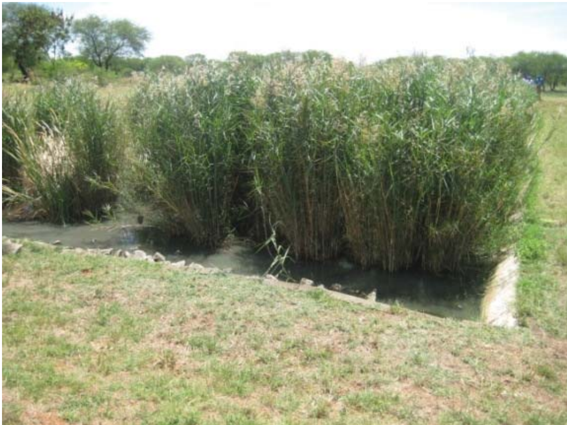
Plate 5: Over-flooding of Shinyanga Prison CW as a result of poor operation and maintenance
